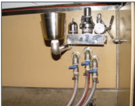
Boiling Pan Double Jacket Water Level Controlling
