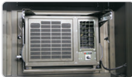
High performance air conditioning unit is used for heating and cooling of the living area. The air conditioner has a maximum cooling capacity of 4.9 kW which is performed as a combination of sensible and latent cooling. The air conditioner can adapt to ambient temperatures from -32° to +60°C.
